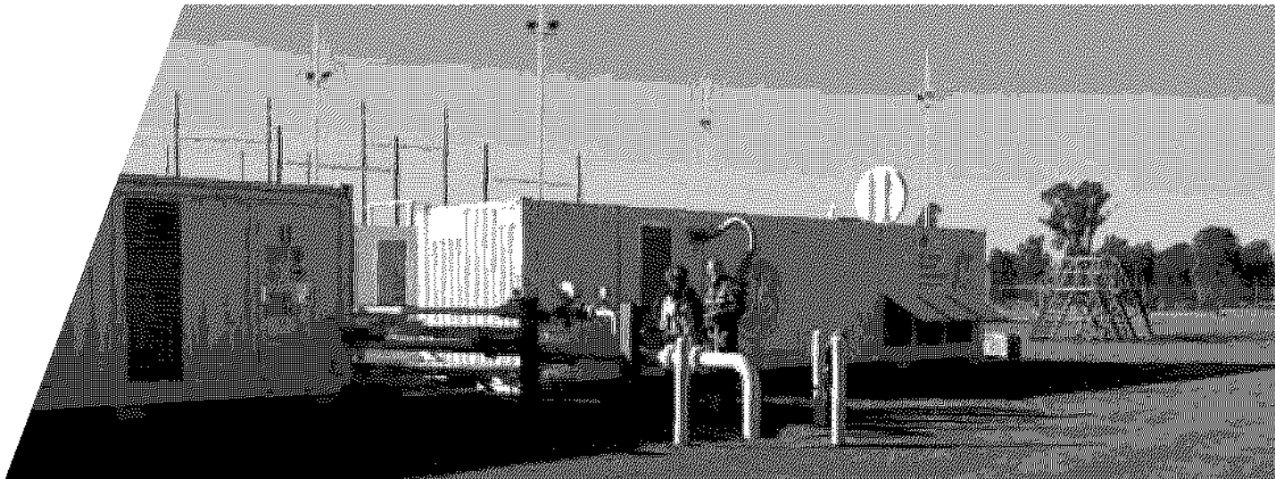
Below: IMW Jenbacher Natural Gas Fired Generator.
