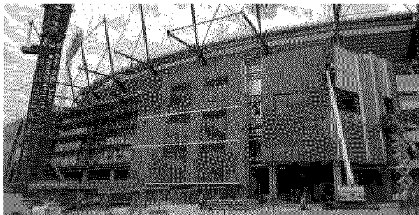
⤴ As part of an extensive redevelopment for the 2006 Commonwealth Games, we installed photovoltaic solar panels on the new members stand entrance at the Melbourne Cricket Ground. More than 15 kilowatts of large commercial panels will generate 10 to 15 megawatt hours of electricity each year and reduce greenhouse gas production by 450 tonnes over the system's life.
