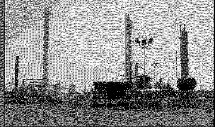
Central processing facilities located at Shefcik 1
