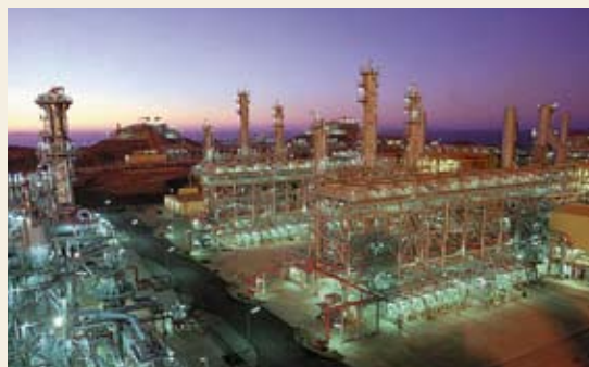
Operations: Over almost two decades, we have established an exemplary LNG capability at the Karratha gas plant, whilst maintaining an excellent safety and environmental record.
