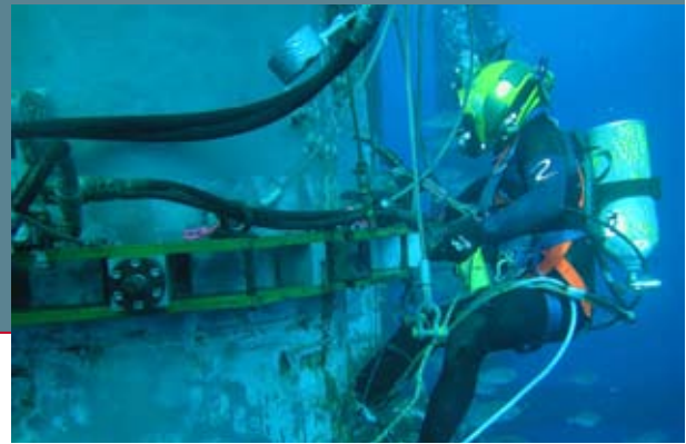
Pipelines: Woodside uses a combination of divers and remotely operated vehicles to check and maintain subsea equipment such as pipelines.
