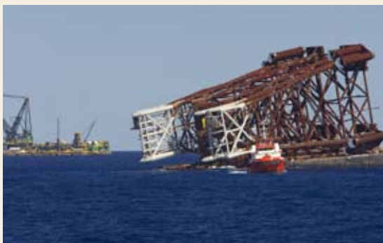
Platforms: The Angel platform was launched from a barge to stand on the seabed. It weighs just over 7,000 tonnes and is over 90 metres high.
