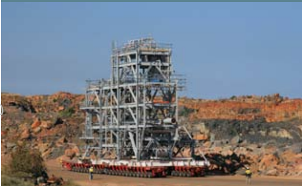
Modular LNG: Having set a new standard in LNG train design and construction, Woodside will use the same approach for Pluto.
