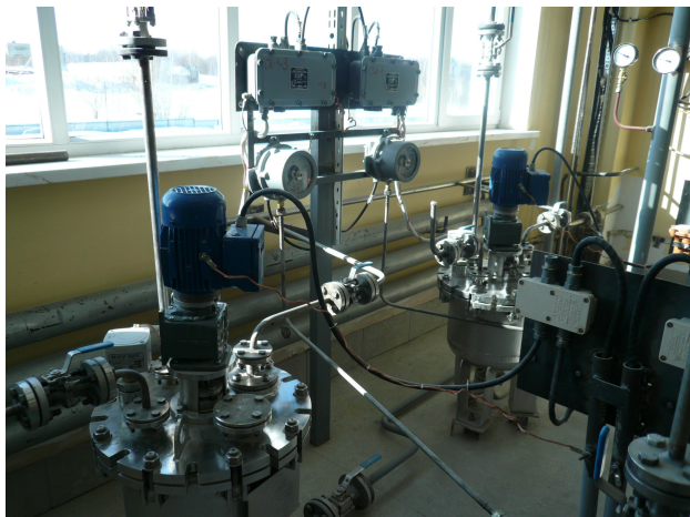
Pipeline and equipment for first and second stage chromatography
