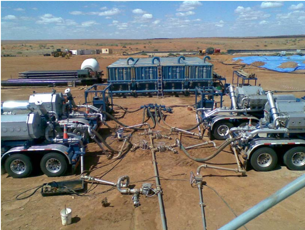
Re-injection pumping array at Habanero 1
