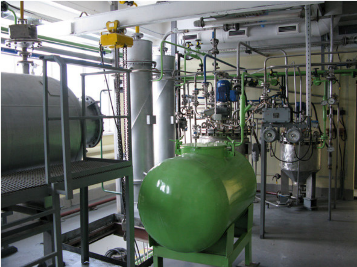
Elements of the Solvent Extraction line
