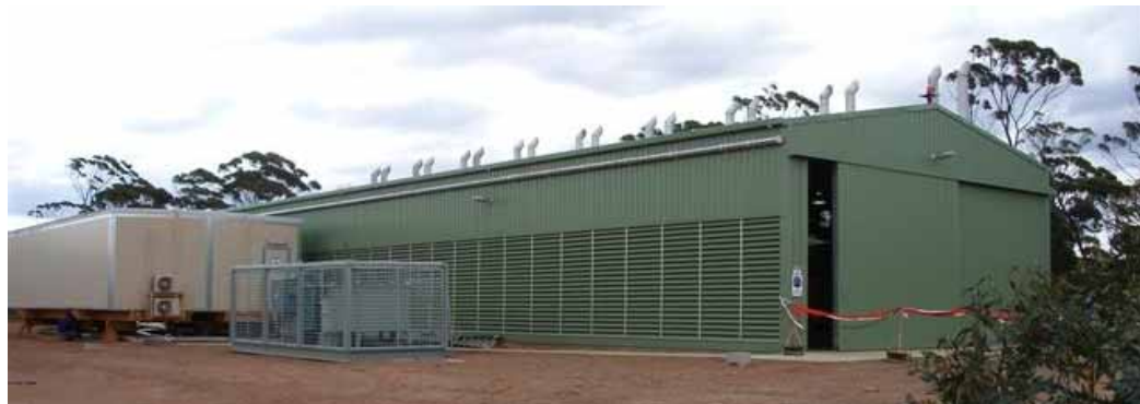
Power station and adjacent switch room
