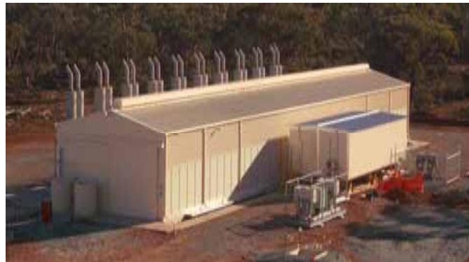
Typical KPS Power Station
