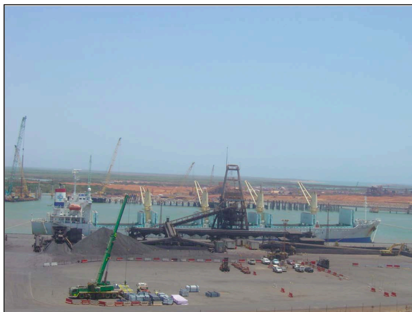
Inaugural shipment of Ant Hill ore being loaded at Port Hedland with new Utah Point berth construction visible across the harbour.
