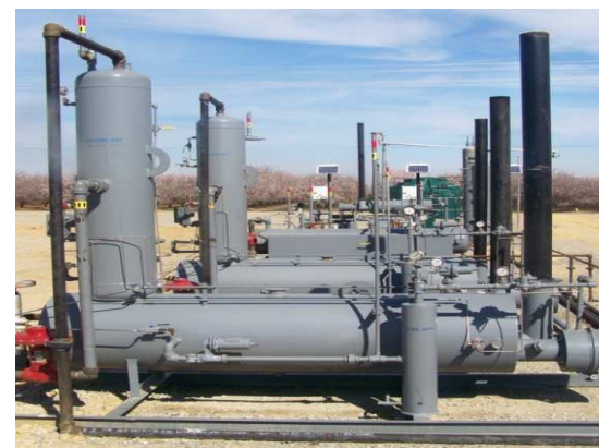
SELH 3 well gas production facility
