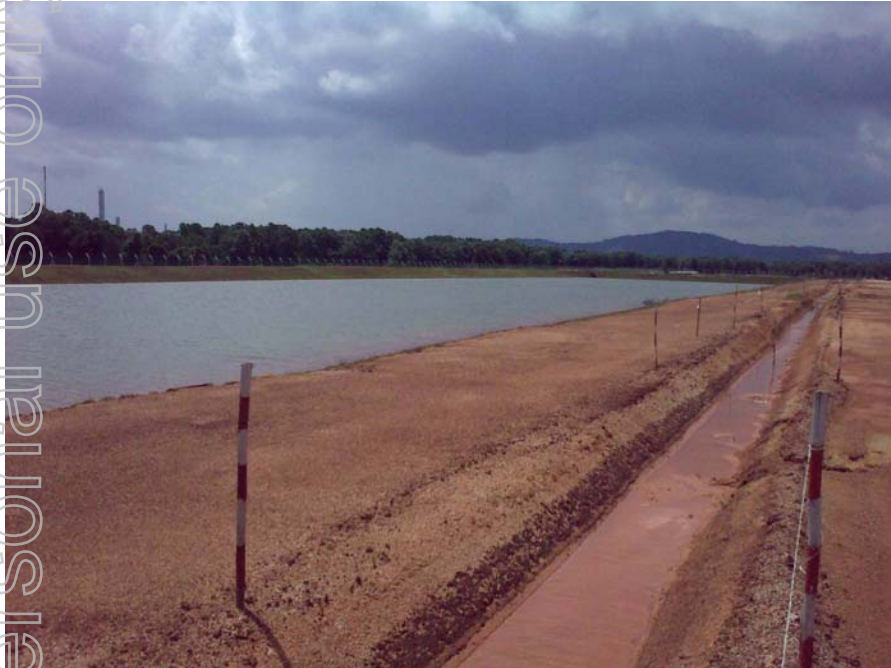
Lynas-constructed stormwater detention pond
