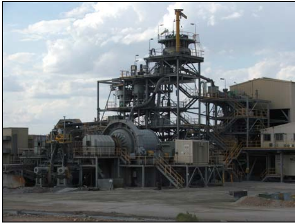
Kanmantoo Project Process Plant
