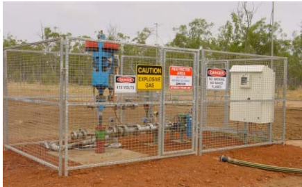
Typical Dart wellhead
