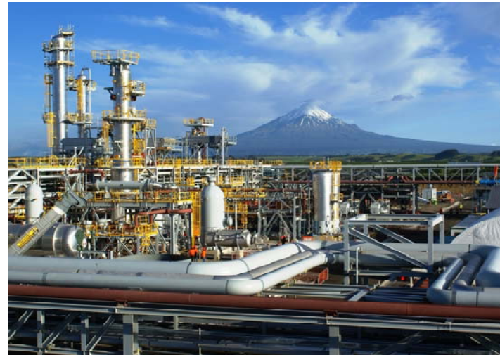
Kupe onshore production facilities
