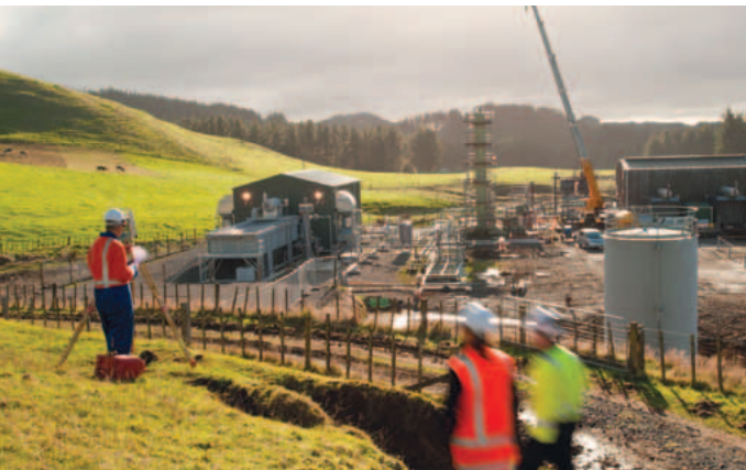
Ahuroa gas storage facility in Taranaki, New Zealand
