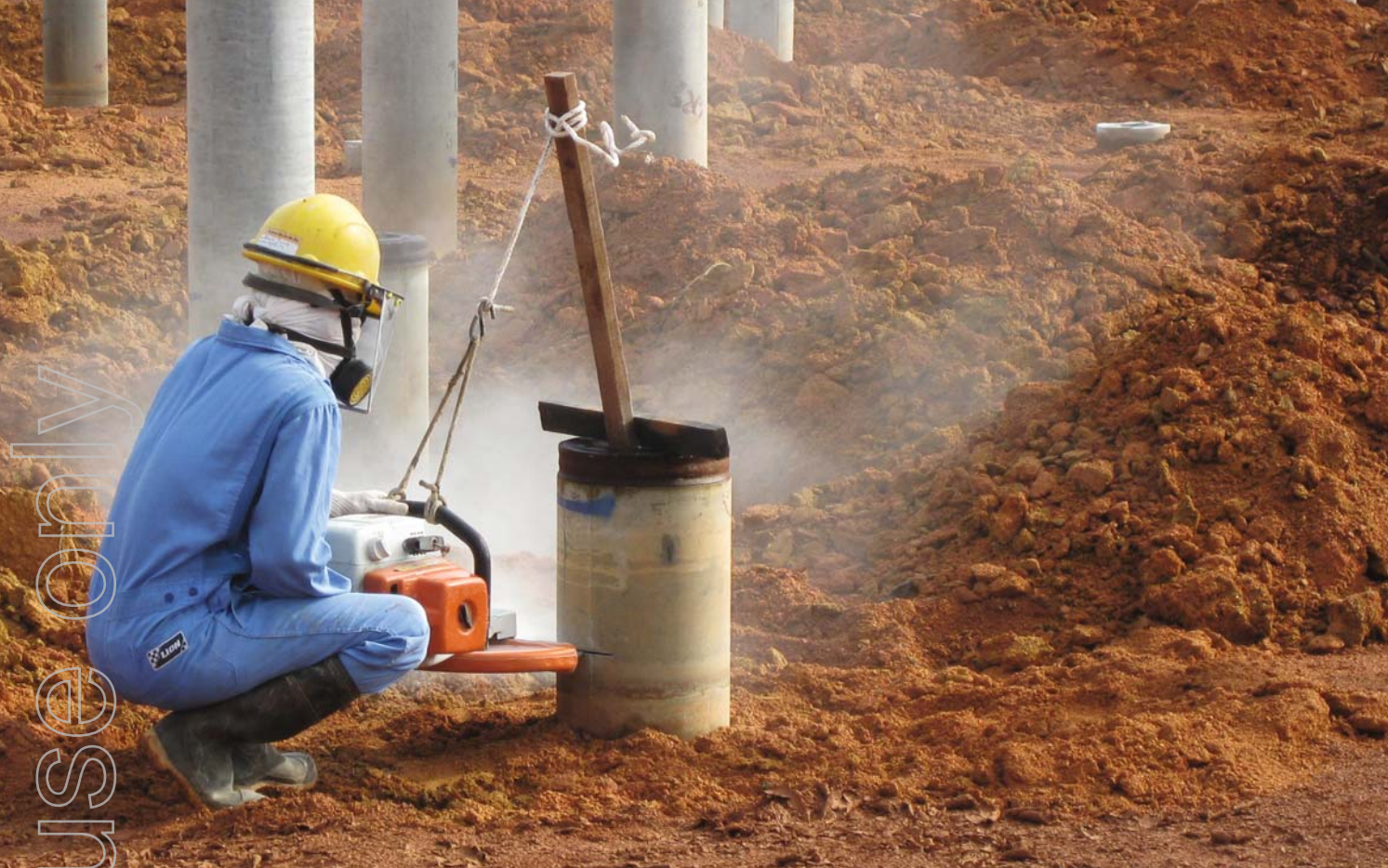
Pile cutting in progress at the Lynas Advanced Materials Plant (LAMP), Malaysia.
