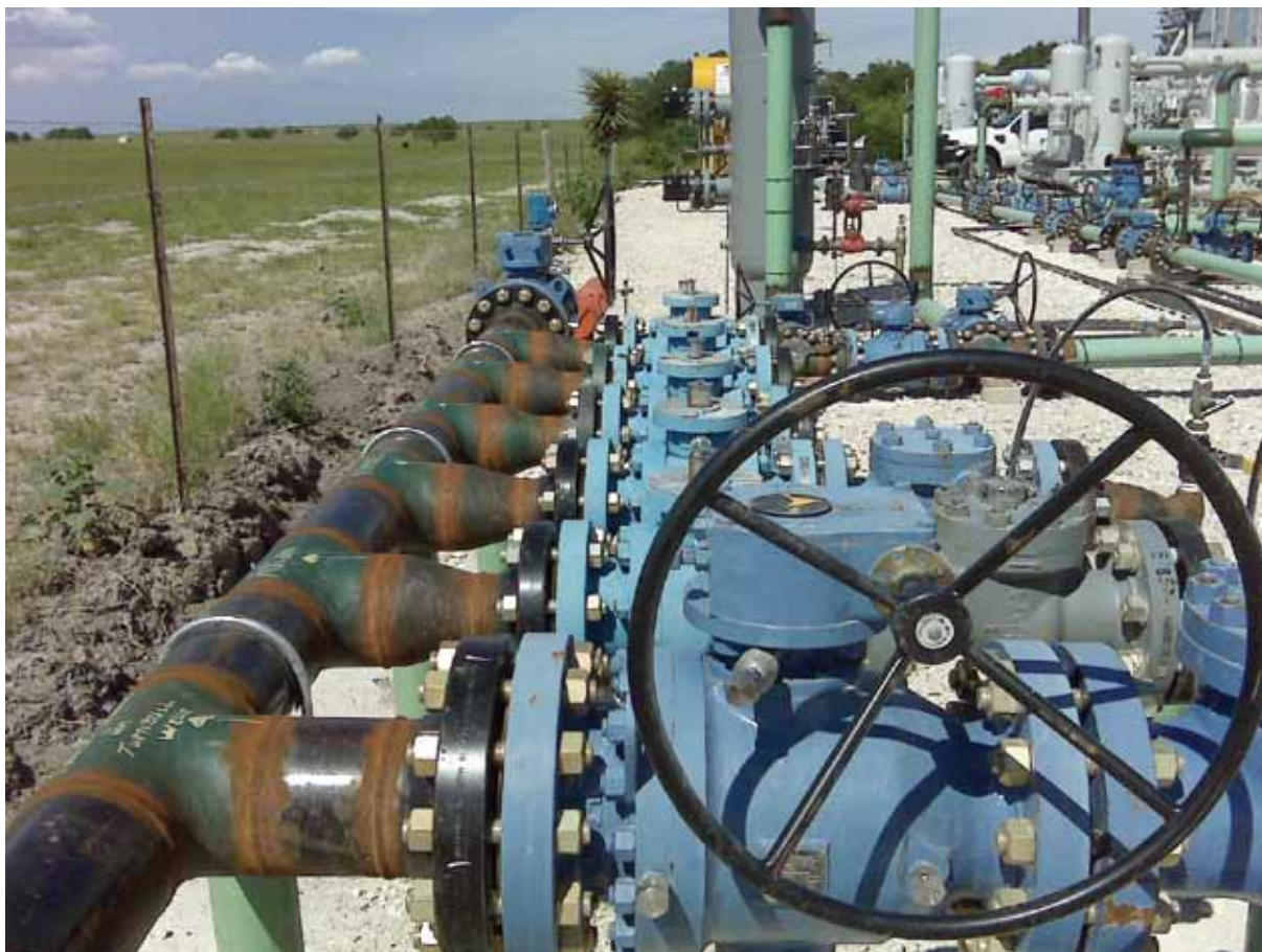
Sugarkane LPG stripping facilities.
