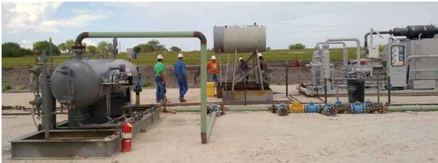
Surface facilities at Sugarkane
