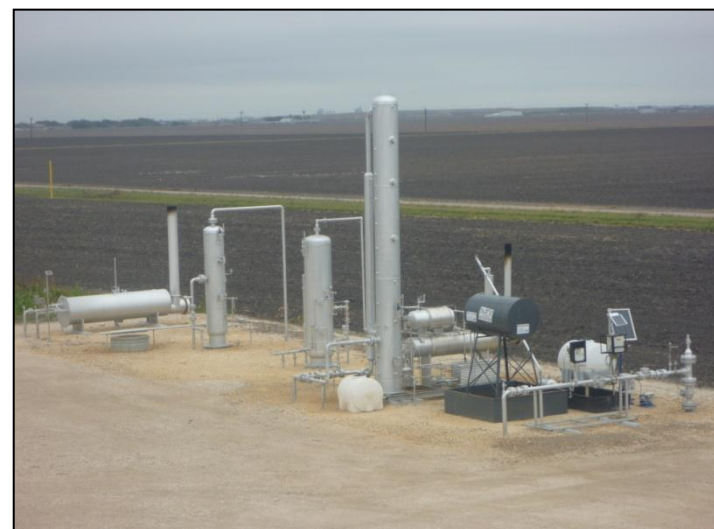
Processing facilities at the Russell Bevly well site
