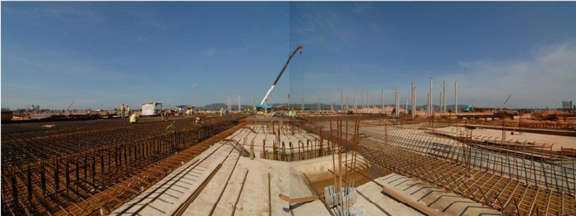
Foundation works and steel reinforcement in place ready for further concrete pours
