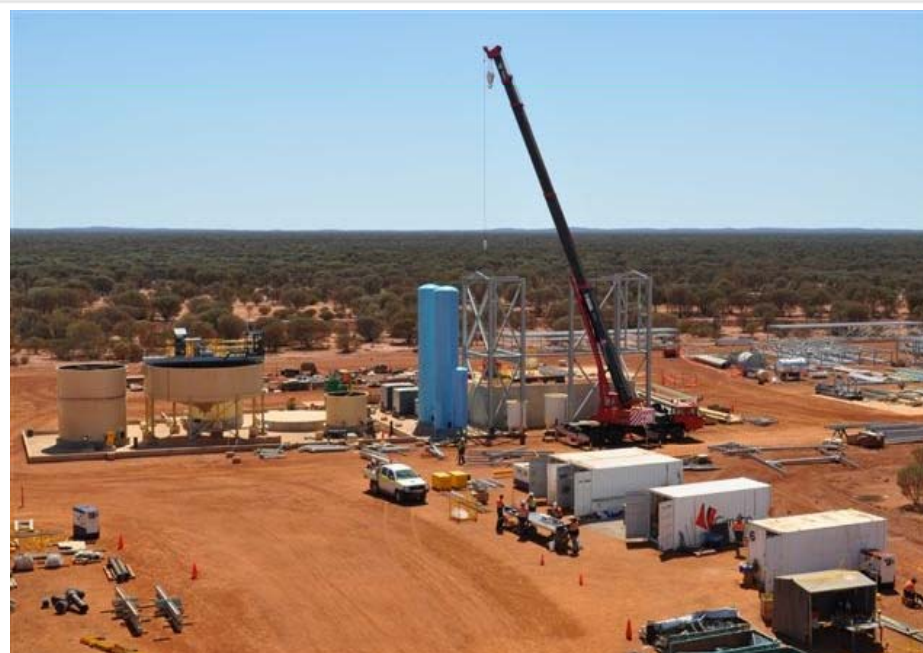
Concentration thickener and packing area
