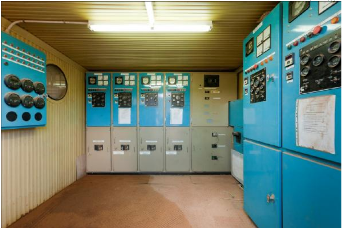
Pic 3 – Gullewa Plant Control Room
