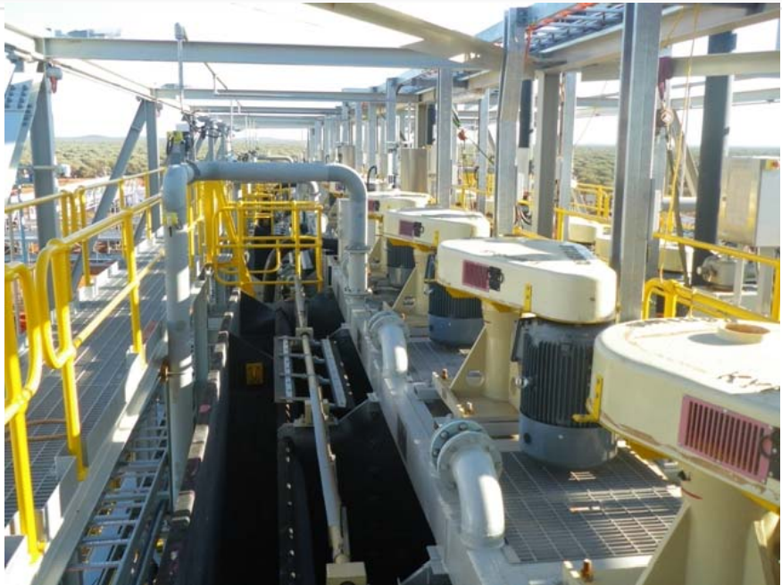
View along top of Flotation Circuit
