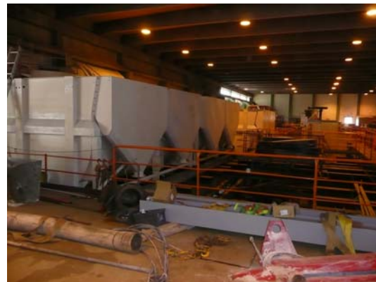
New float cells installed in mill hall
