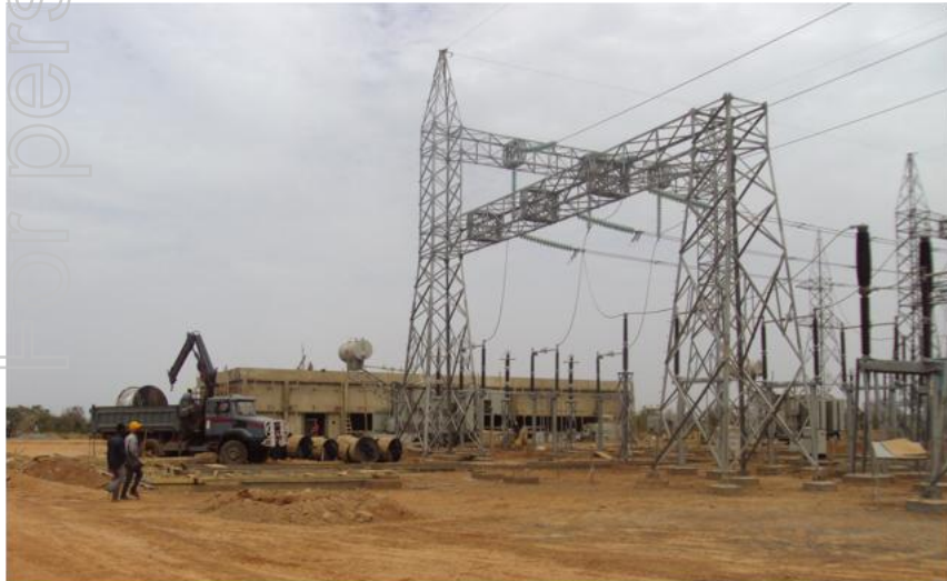
Sikasso Substation Feb 2011
