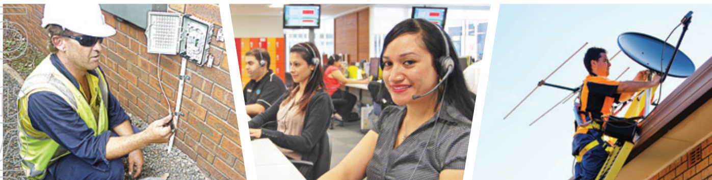
Contracting Solutions (above) From left: Providing Fibre to the home; Call Centre Representatives; FOXTEL installation
