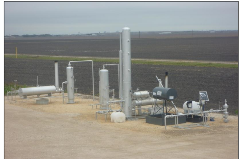
Processing Facilities at the Russell Bevly Well Site
