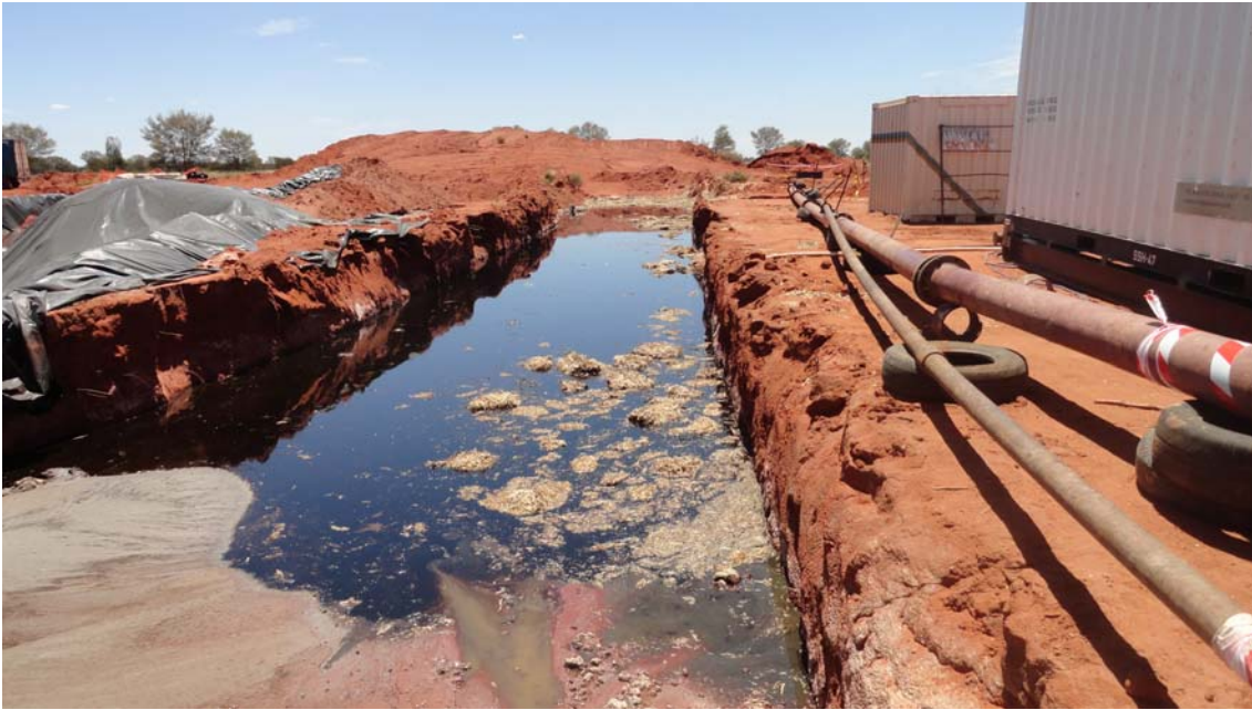
Layer of oil on surface of sump during drilling. This has now been skimmed off and stored in environmentally safe containers for later disposal.
