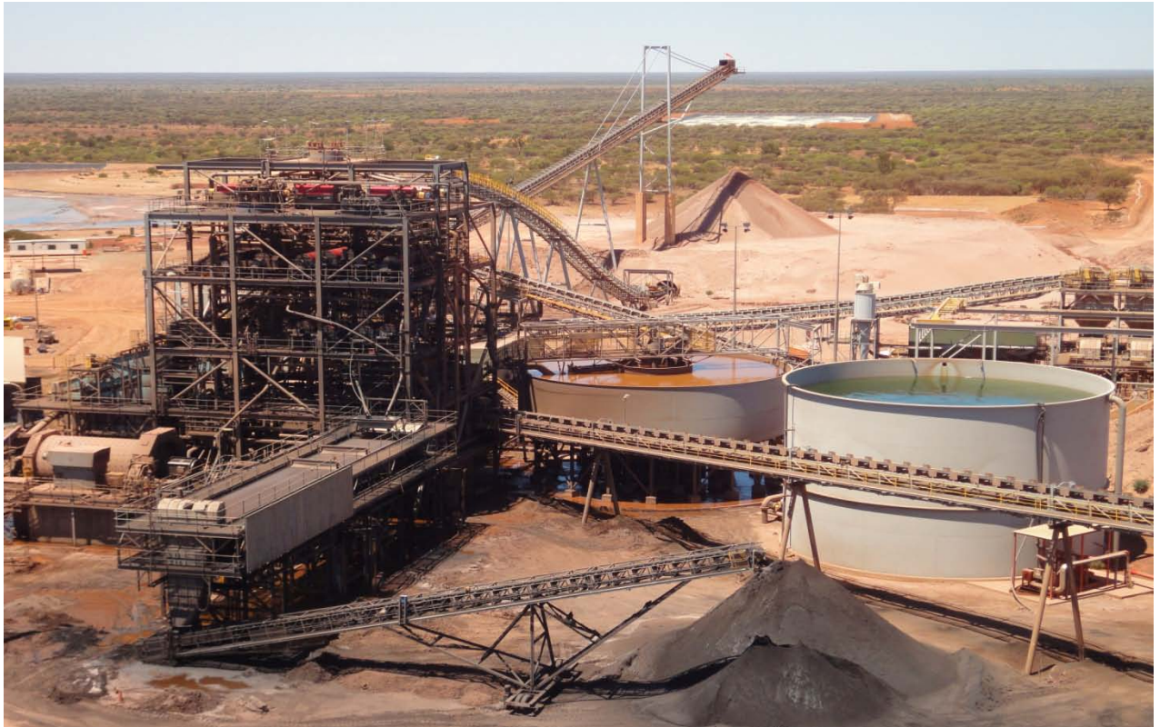
Crushing, milling and beneficiation circuit at Windimurra with magnetite concentrate product in foreground
