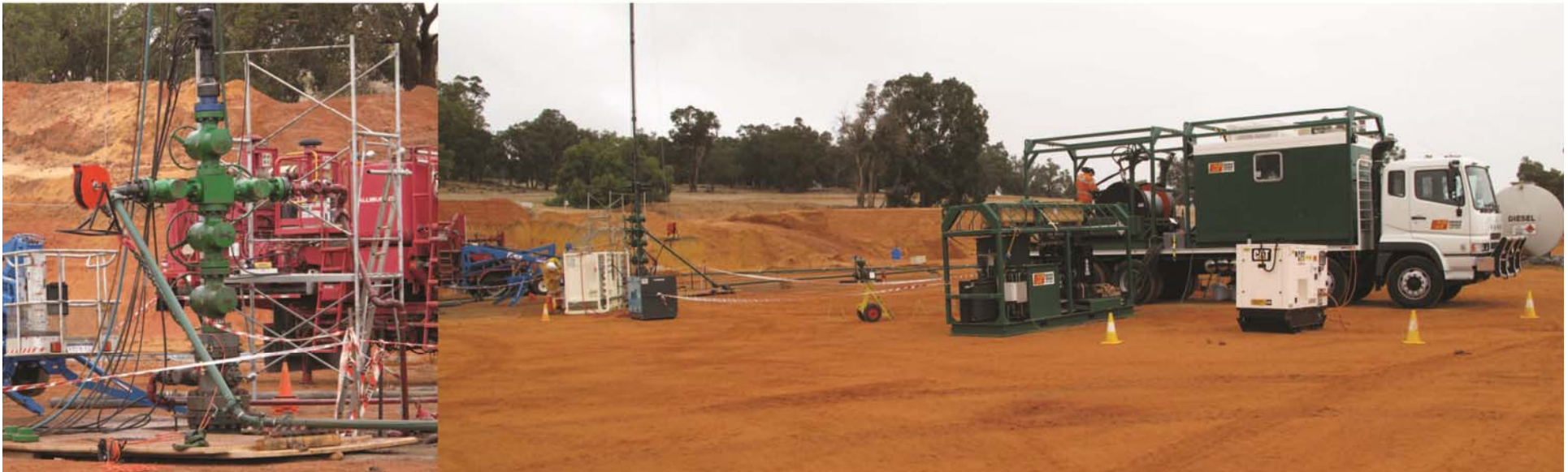
Perforating Gingin West-1 with new electric logging company, Crocker Trucker Energy Services Pty Ltd, with wireline through tubing guns.
