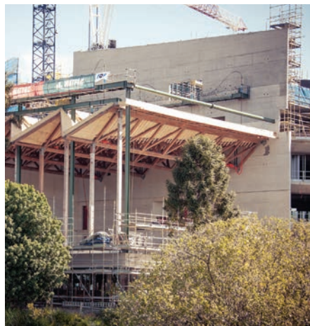
Watpac recently successfully completed lifting and installing a 200 tonne roof on UQ's Advanced Engineering Building
