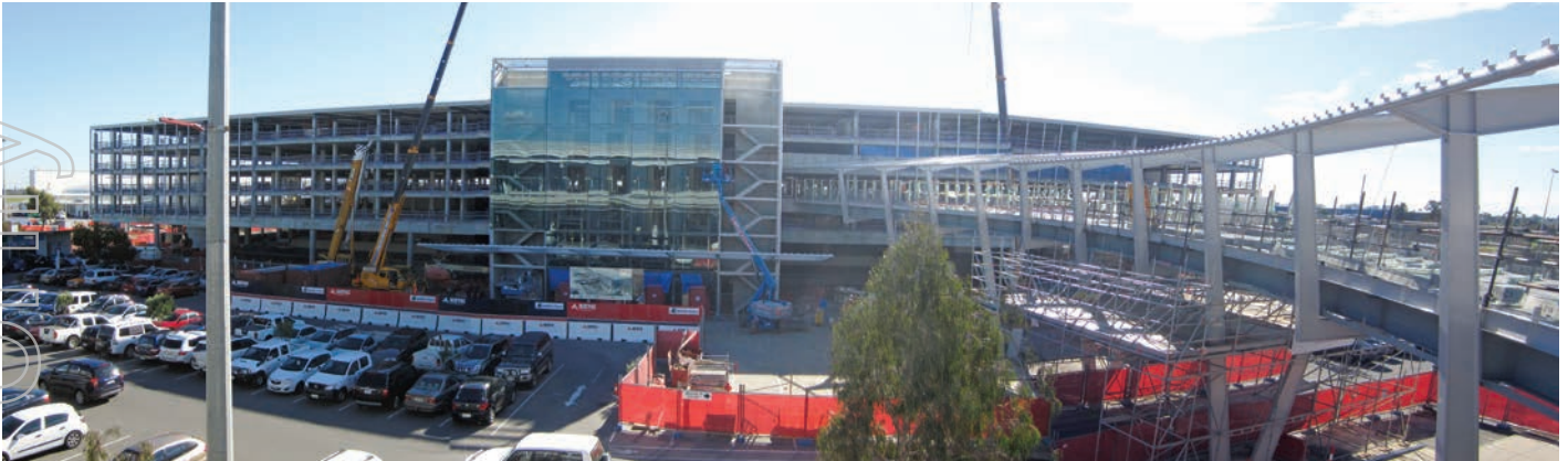
Construction on Adelaide Airport's new multi-level car park will be completed later this year
