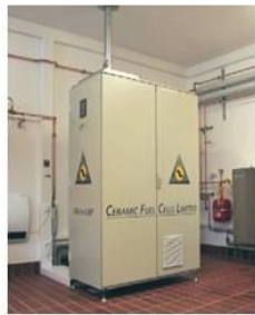
CHP-2 and NetGen
