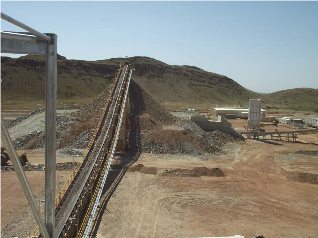
Crushed Ore on CV01 to the Reclaim Stockpile
