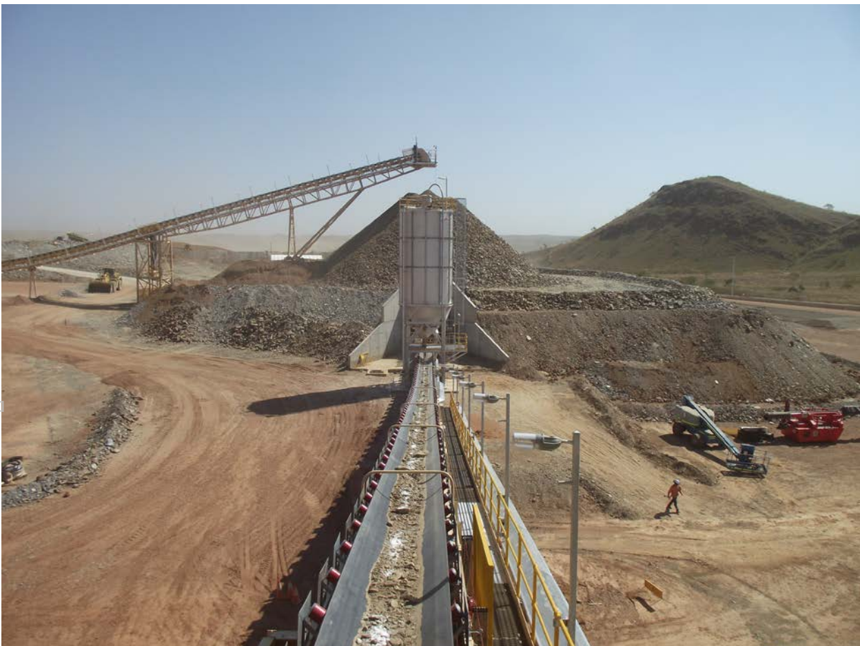
CV2 to Mill – Crushed Ore and Lime to Mill. Crushed Ore Stockpile-Background
