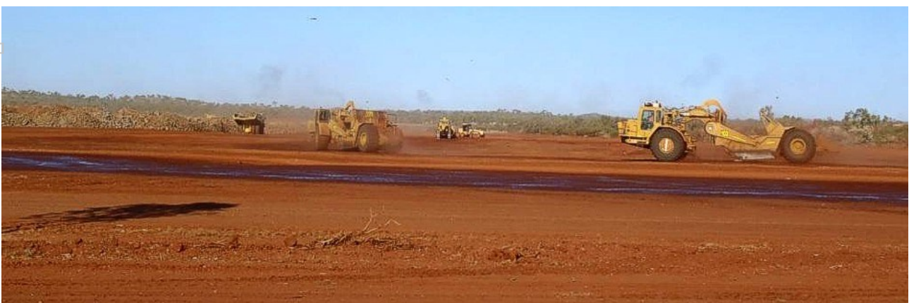
Figure 3: Scrapers (foreground), dump trucks (left), dozers, graders and water-trucks (middle backgoud), constructing the main Water Storage Facility at Rocklands, primarily designed to provide water to the Rocklands Process Plant.
