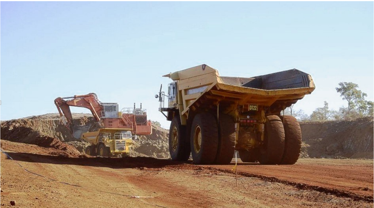
Figure 1: Excavation of the diversion channel, removing material from the second shot of the project. Dump trucks wait in line as each is loaded by the Hitachi 1900 Excavator. All Equipment is 100% owned by CuDeco.
