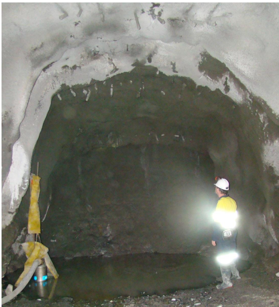
End of Union Hill Decline with spiling bars (steel rods) and shotcrete covered concrete arches
