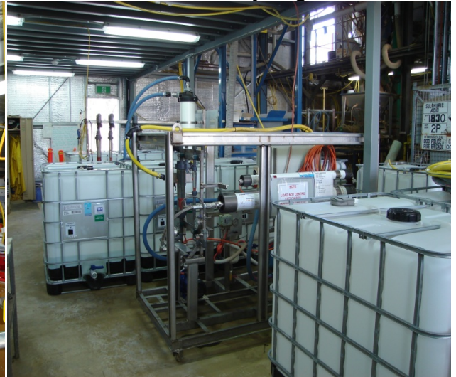
Reverse osmosis water recycling DPP
