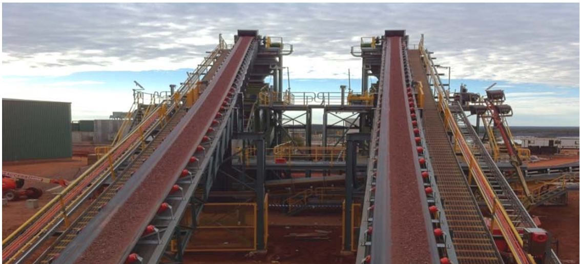
Crushed ore enters the new screening plant commissioned at the start of the quarter
