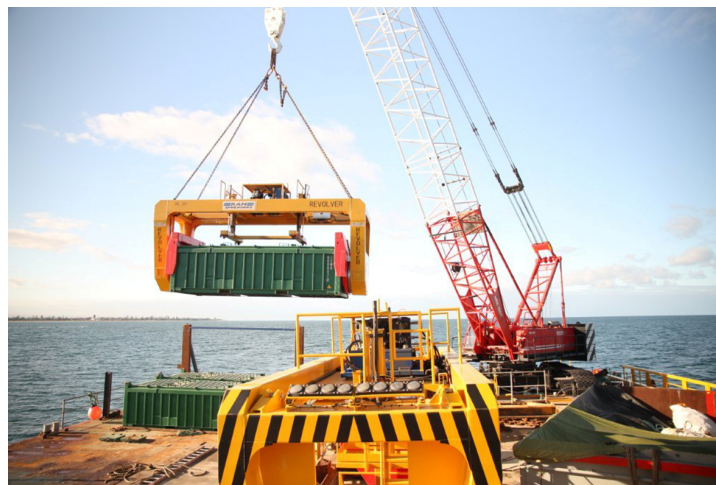
Container being lifted from dumb barge by use of floating crane and IronClad’s custom built rotainer
