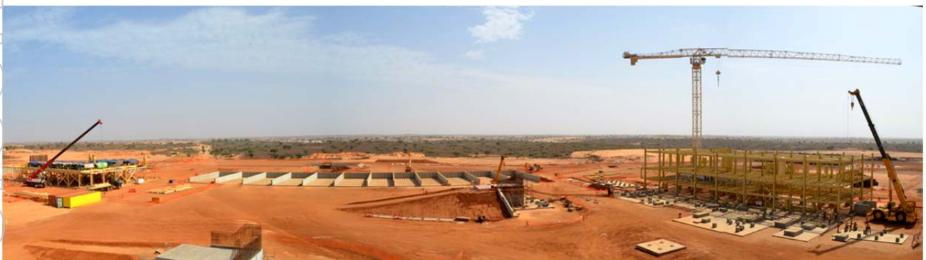
Construction at the MSP - wet mill (left), intermediate zircon storage (centre) & dry mill (right)
