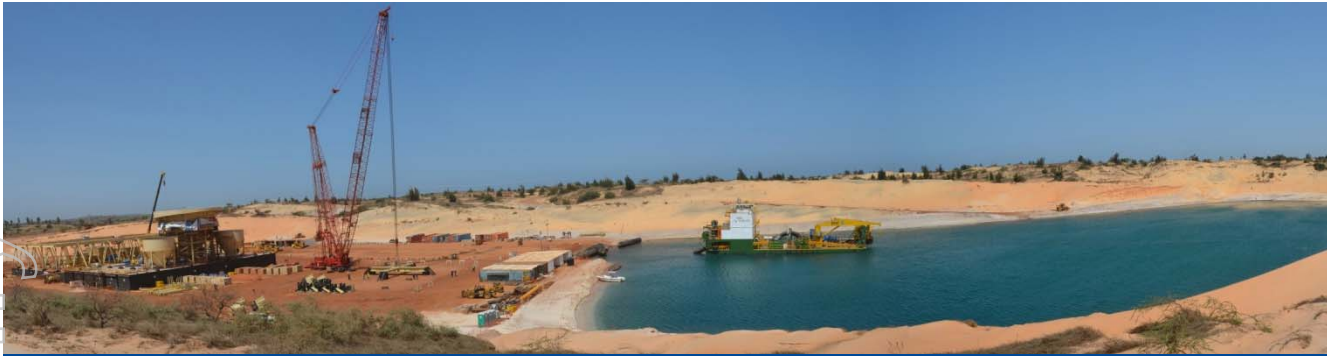
After launch, the dredge floats on the start-up pond, while construction of the WCP continues (left)
