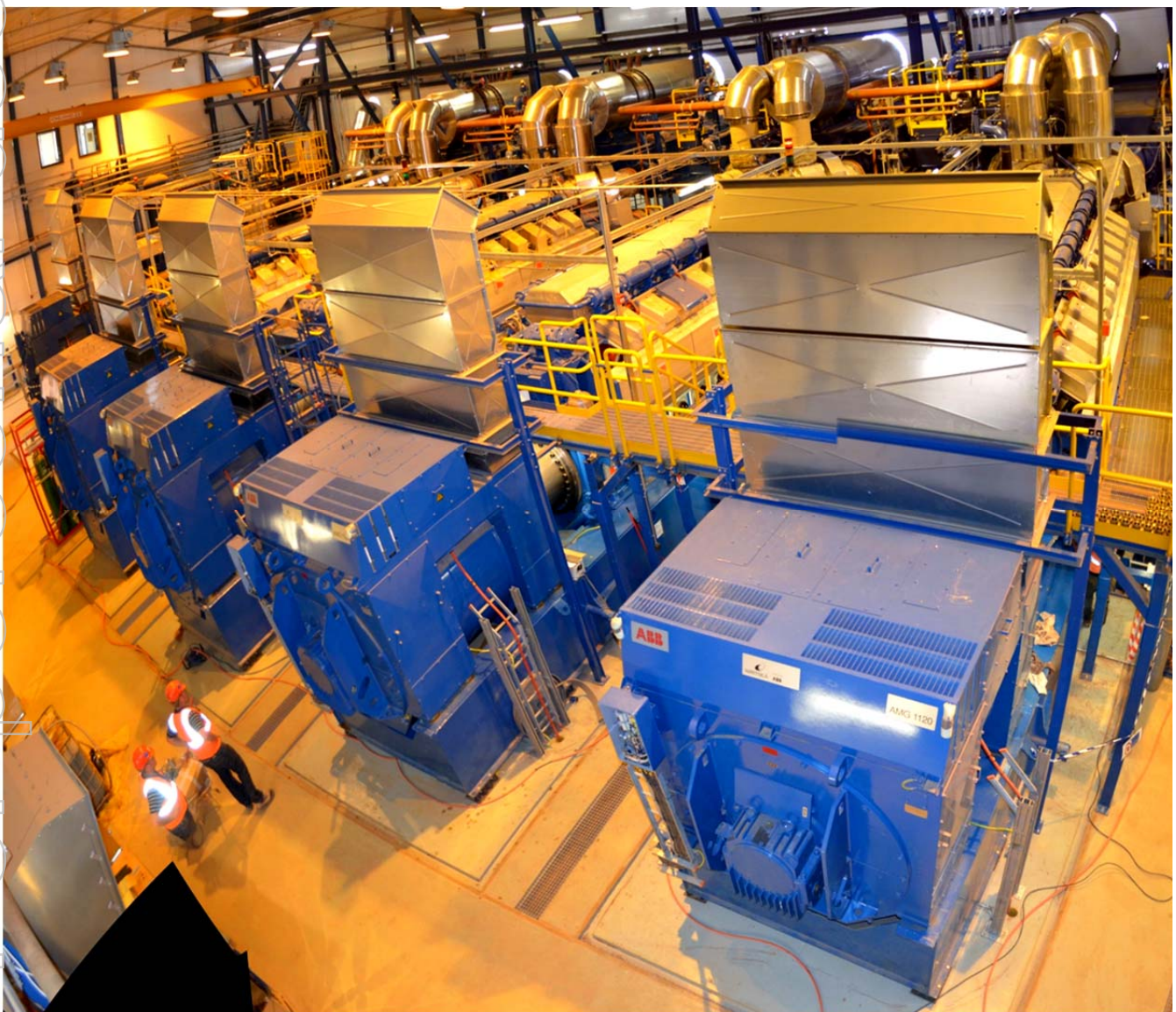
Inside the newly-built power station
