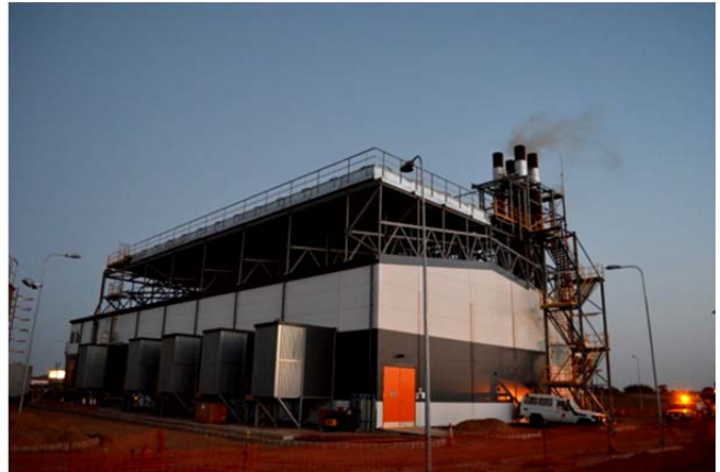
First engine started at the power station
