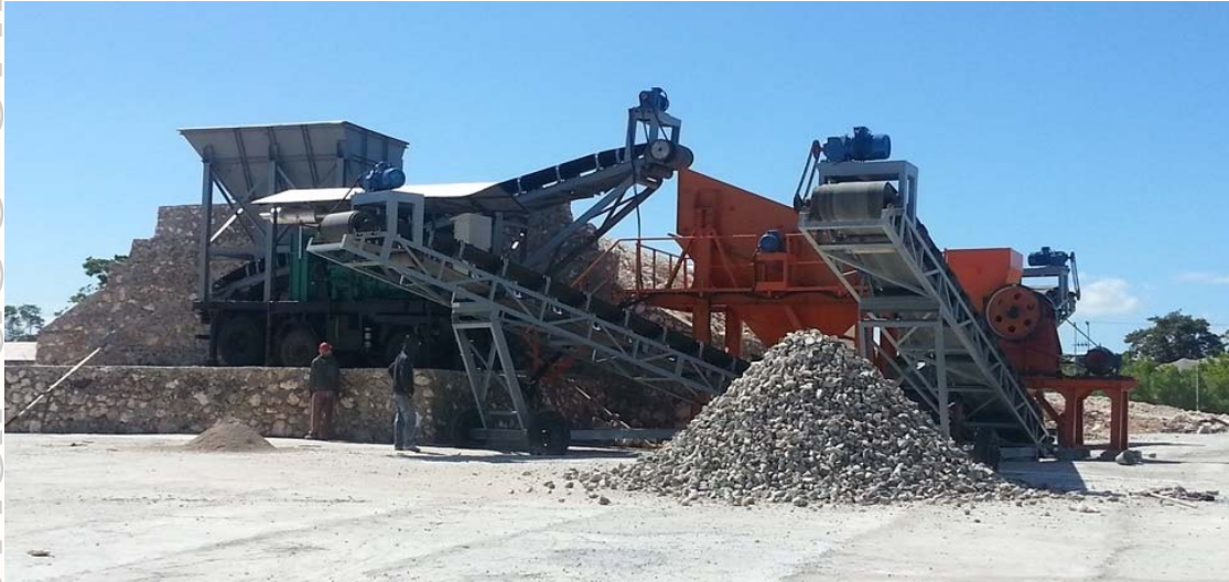
Dry Commissioning Kupang Process Plant - 30 Jun13
