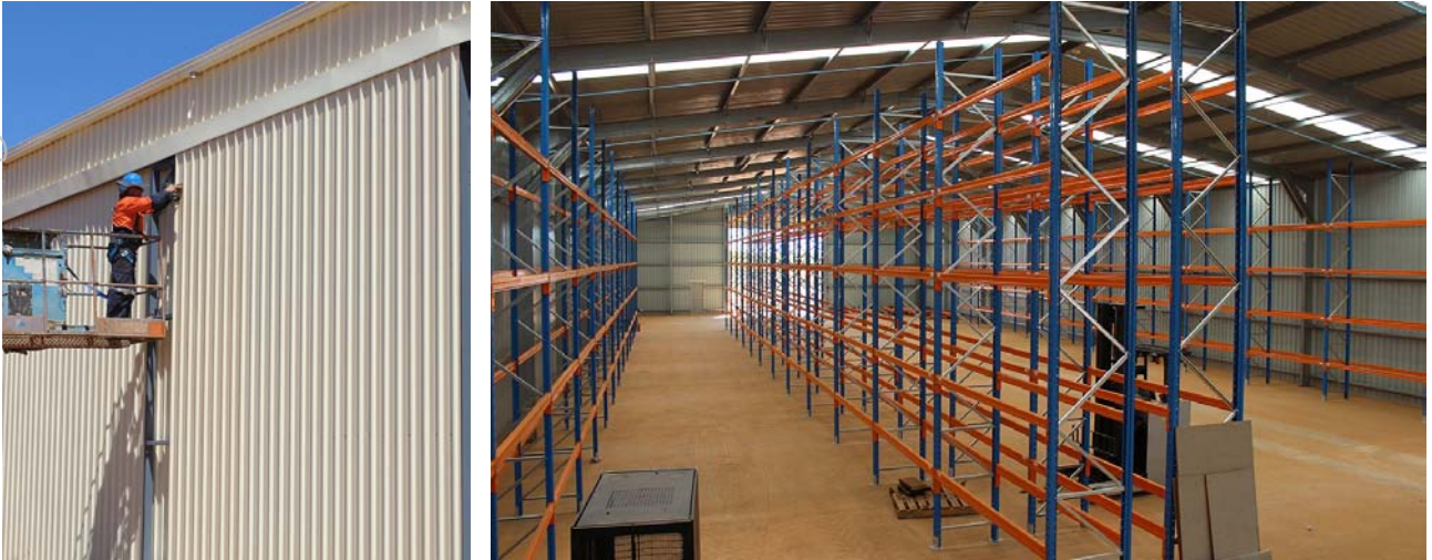
Figure 15: Final touches to the new Stores Warehouse, which also includes a data centre and offices
