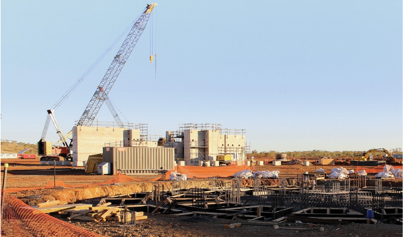
Figure 1: Formwork for gravity thickener in foreground, and completed concrete work at Ball Mill housing in background.
