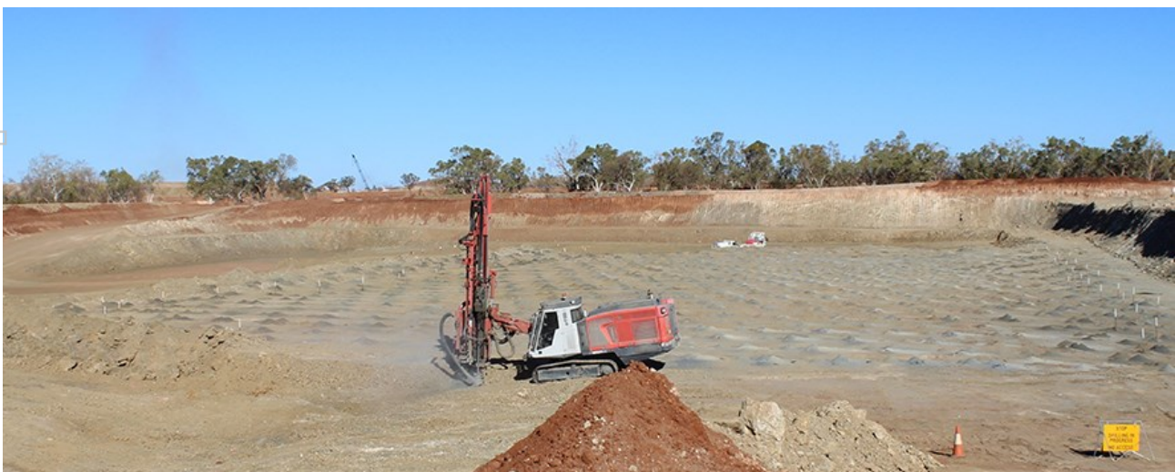
Figure 19: Blast-hole drilling has commenced in waste areas adjacent to the main ore zones at Las Minerale - ore areas are still free-dig at this stage.
