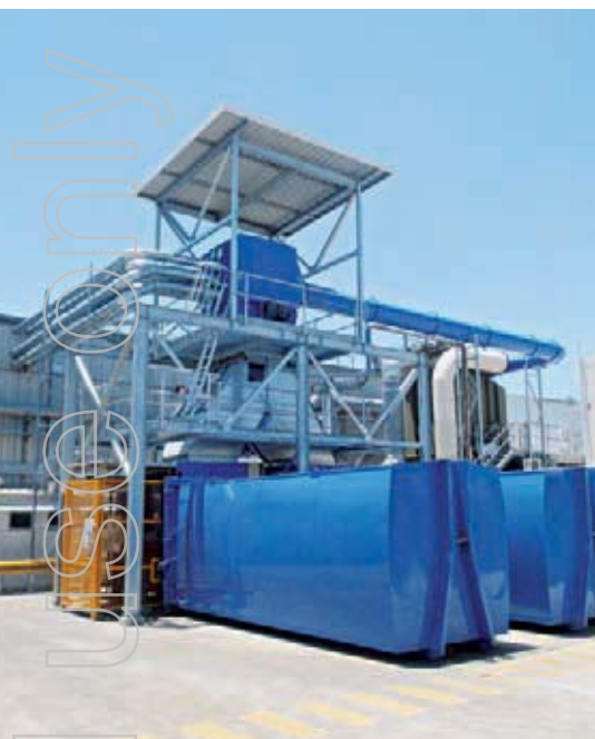
Above A new variable speed extraction system and compactor replaces the inefficient constant velocity push-pull paper waste extraction system. This has reduced electricity consumption, reduced environmental pollution from loose shredded paper, increased recycling rates and increased reliability.
