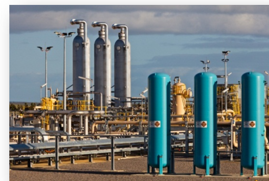
Mondarra Gas Storage Facility
