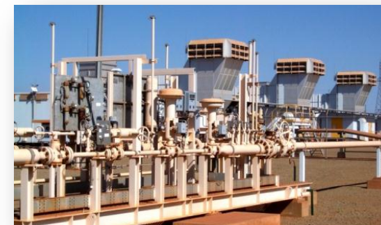
Regulator skid at Newman Power Station
