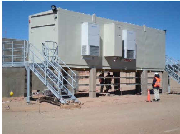
Electrical control room
