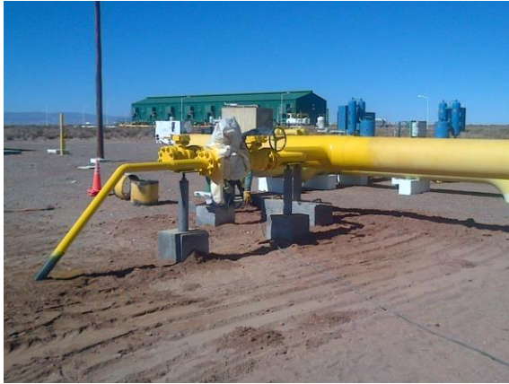
Gas Atacama branch line connection
