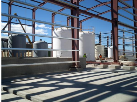
Lithium carbonate plant
