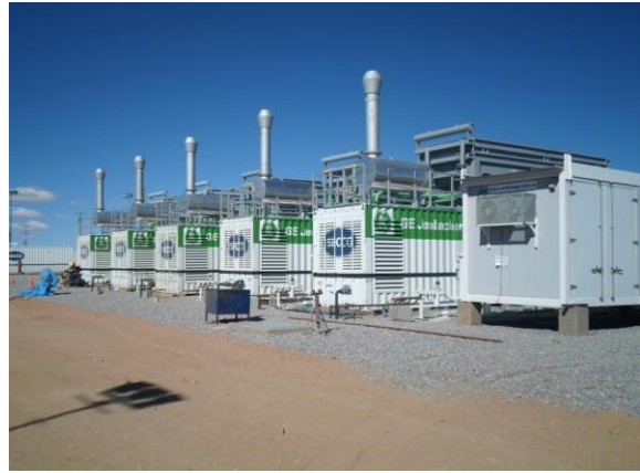
Power generation station
