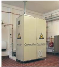
CHP-2 and NetGen
