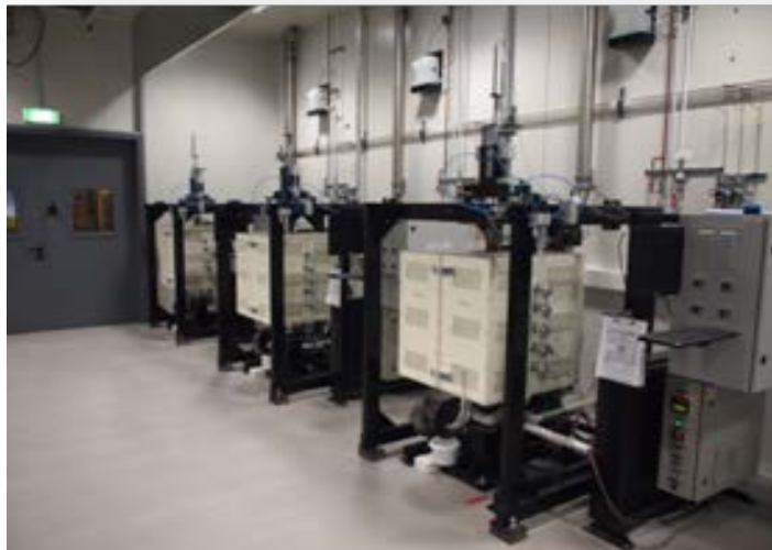
Single stack furnaces
