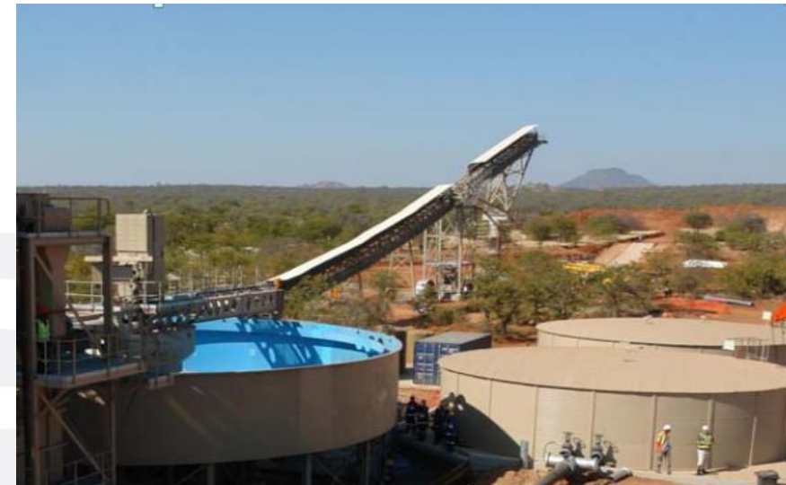
Thickener and product stockpile
