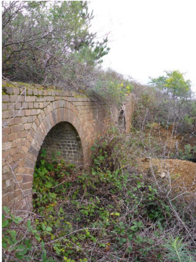
Figure 3 Extract from Heritage survey "Plate 52", remnants of brick calcining kiln looking south.
