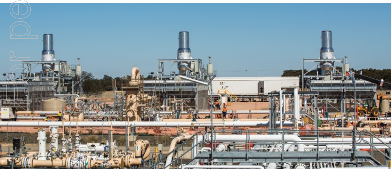
Three new Solar Mars 90 compressors installed at Wallumbilla, adding to six existing compressor units.
