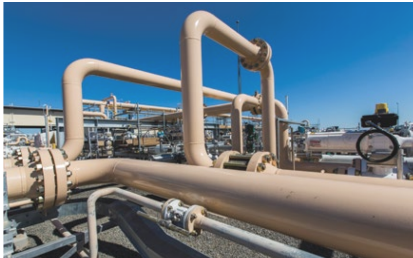
Modification of the SWQP pipeline at Wallumbilla to allow bi-directional flow capability.
