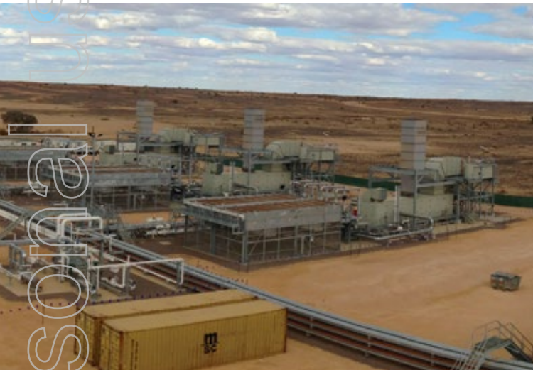
Expanded compression capacity at Moomba with the installation of 3 new Solar Mars 90 compressors.
