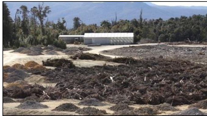
Dec 2013, Topsoil and vegetative matter ready for final placement to support re-growth
