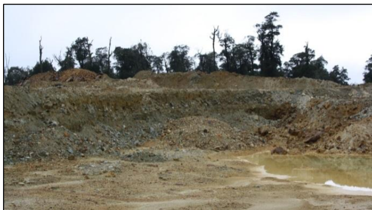
Aug 2013, Prior to commencing the rehabilitation of the Settlement Dam waste stockpile
