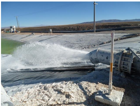
Pumping of brine to evaporation pond
