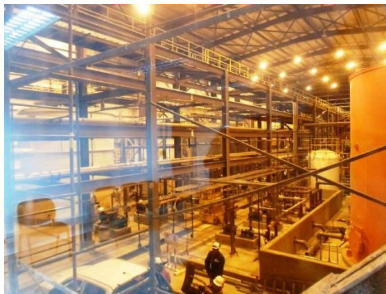
Inside the lithium carbonate building
