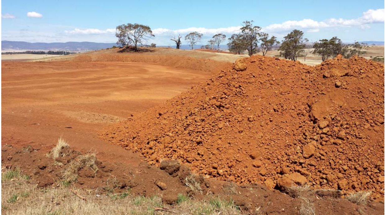
Figure 6: Stockpiled bauxite at the screening site. Screening plant arrived at site 29 January to commence screening trials on 30 January. A second bauxite pit workings is in the distance (top centre). Because this second pit is high grade, it will be screened once the screening process has been optimised.
