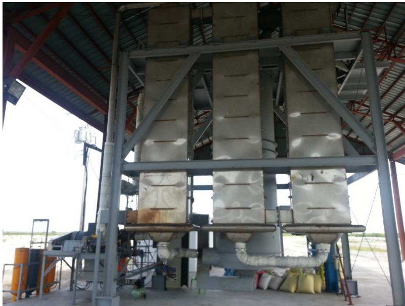
Indirectly Fired Gas Turbine (IFGT)
